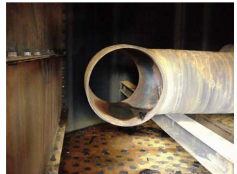
Recovery column feed line
