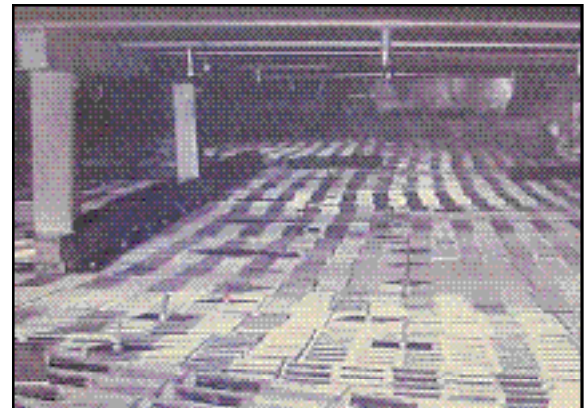
Figure 5 Clean trays in a large vacuum tower after chemical cleaning
